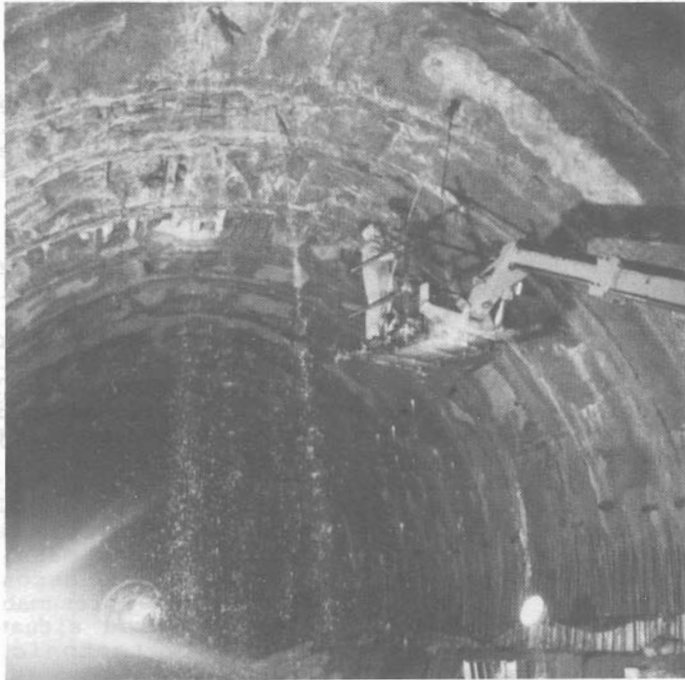
Photo 1: Example of heavy water inflow into Mompantero tunnel
