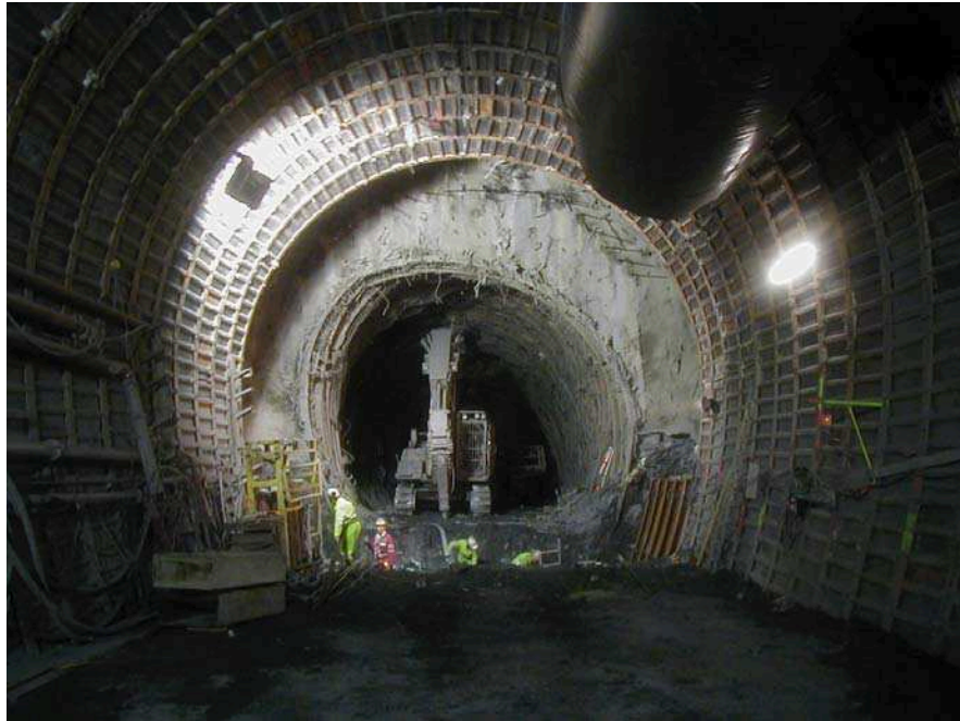
Fig. 3.2: Very severe squeezing behaviour in the S.Martin La Porte adit to the base tunnel of the new railway link Turin-Lyon (→case-history ch1): up to more than 2m of diametral convergence with consequent necessity of tunnel re-shaping (Photo: courtesy of J. Piraud (Antea)).
