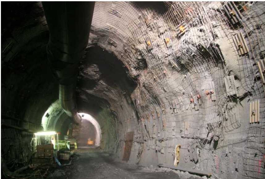
Figure 18. Deformations of the excavation contour of SMLP adit: see Figure 17 for comparison.
