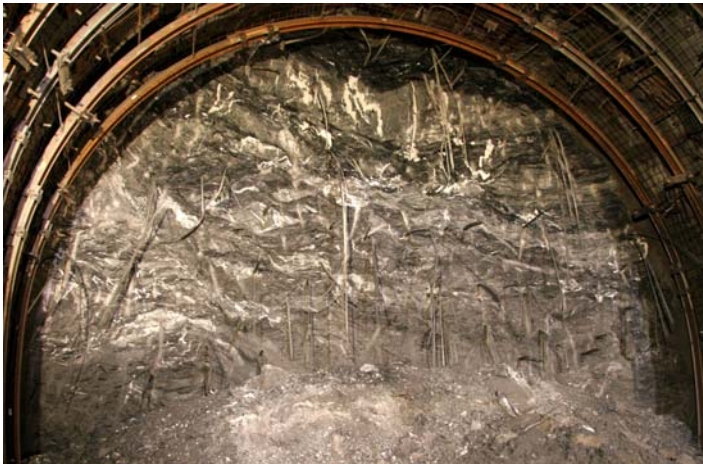
Figure 2. Example of appearance of the graphitic schists of Houiller at the tunnel face.
